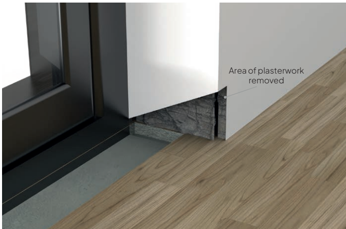
Relieve the plasterwork, allow enough room for the tectite to fit flush to the wall.
