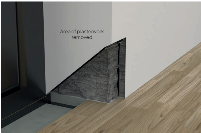
Relieve the plasterwork, allow enough room for the tectite to fit flush to the wall.
